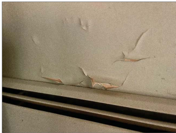
Photo 13 - Water damaged drywall and blistering paint in the moira room (Location 10).
