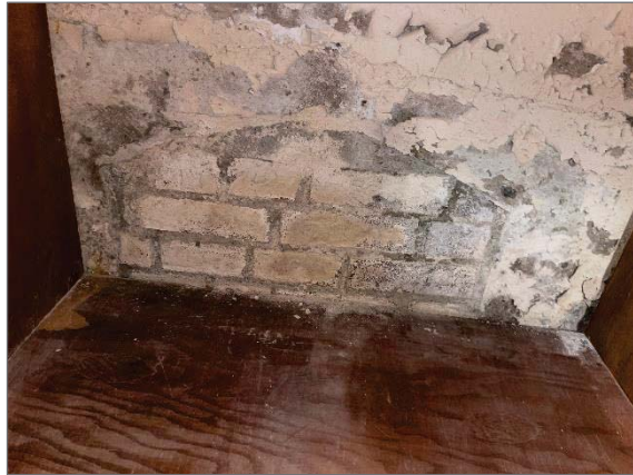
Photo 15 - Efflorescence, deteriorated paint and mortar on masonry foundation wall and mould growth on wood shelving in a storage room (Location 22).
