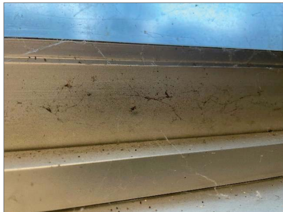
Photo 10 - Mould growth on the metal window frames in the Quinte Room (Location 9).
