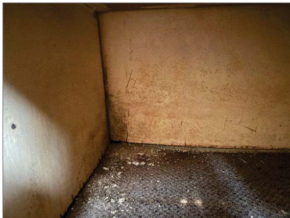
Photo 9 - Mould growth on the drywall wall in the closet of the Quinte Room (Location 9).
