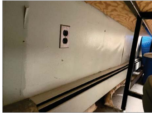
Photo 12 - Water damaged drywall and blistering paint in the moira room (Location 10).
