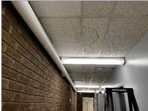
Photo 16 - Water-stained ceiling tiles in the north corridor (Location 8).
