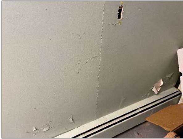
Photo 11 - Water damaged drywall and blistering paint in the quinte room (Location 9).
