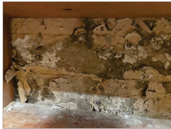
Photo 14 - Efflorescence, deteriorated paint and mortar on masonry foundation wall and mould growth on wood shelving in a storage room (Location 22).
