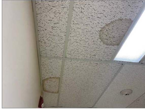
Photo 6 - Water stained ceiling tiles in the west corridor (Location 5).
