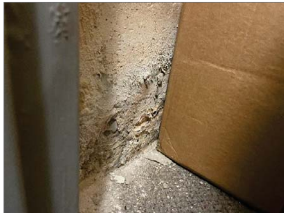
Photo 8 - Efflorescence and deteriorated paint and mortar on masonry foundation wall in the closet of the Quinte Room (Location 9).
